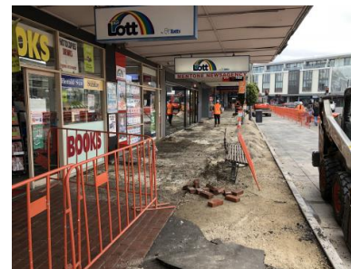
Como Parade West, Mentone Shopping Centre – west side footpath replacement during construction
