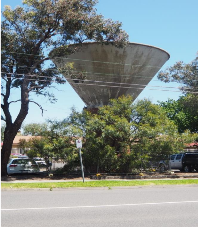
Mordialloc Railway Water Tower (HO92). Built circa 1910. Used for replenishing steam trains. (Source: RBA, November 2022)
