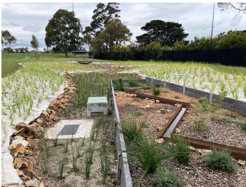
Stormwater treatment installed at Keeley Park, Clayton South (2023)
