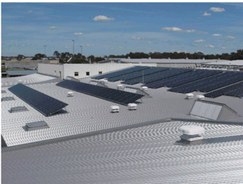
Parkdale Hub solar system, Warren Road.
