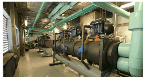
Efficient chiller at the 1230 Nepean Hwy, Cheltenham Municipal Office.
